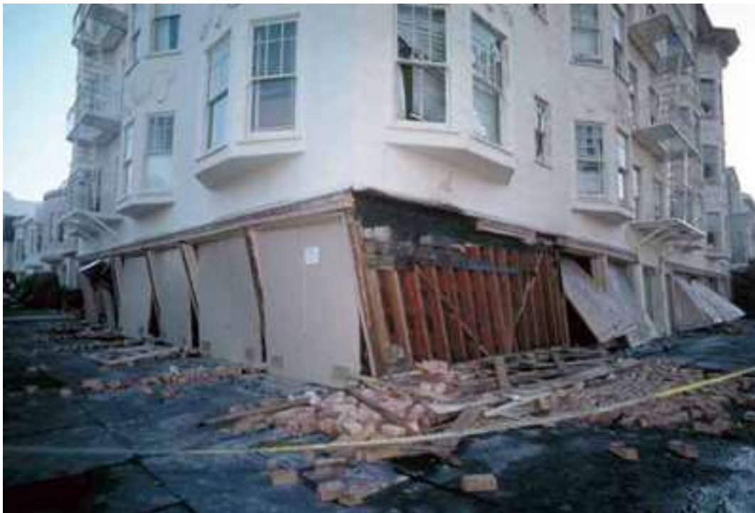
Figure 7-16. Soft-Story Damage from Earthquake
