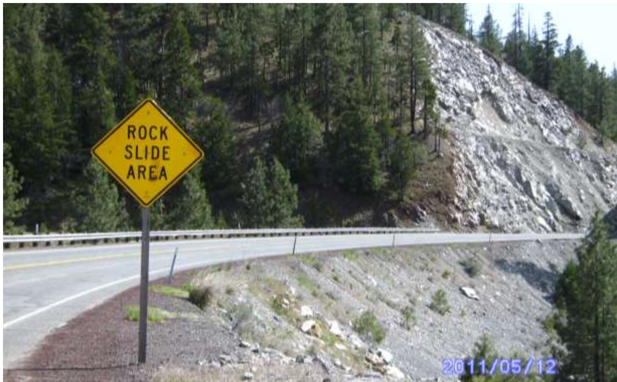
Figure 13-5. California State Route 3—Fort Jones Road Rock Slide Area
